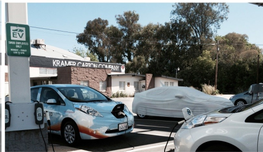
ELECTRIC VEHICLE CHARGING STATION
